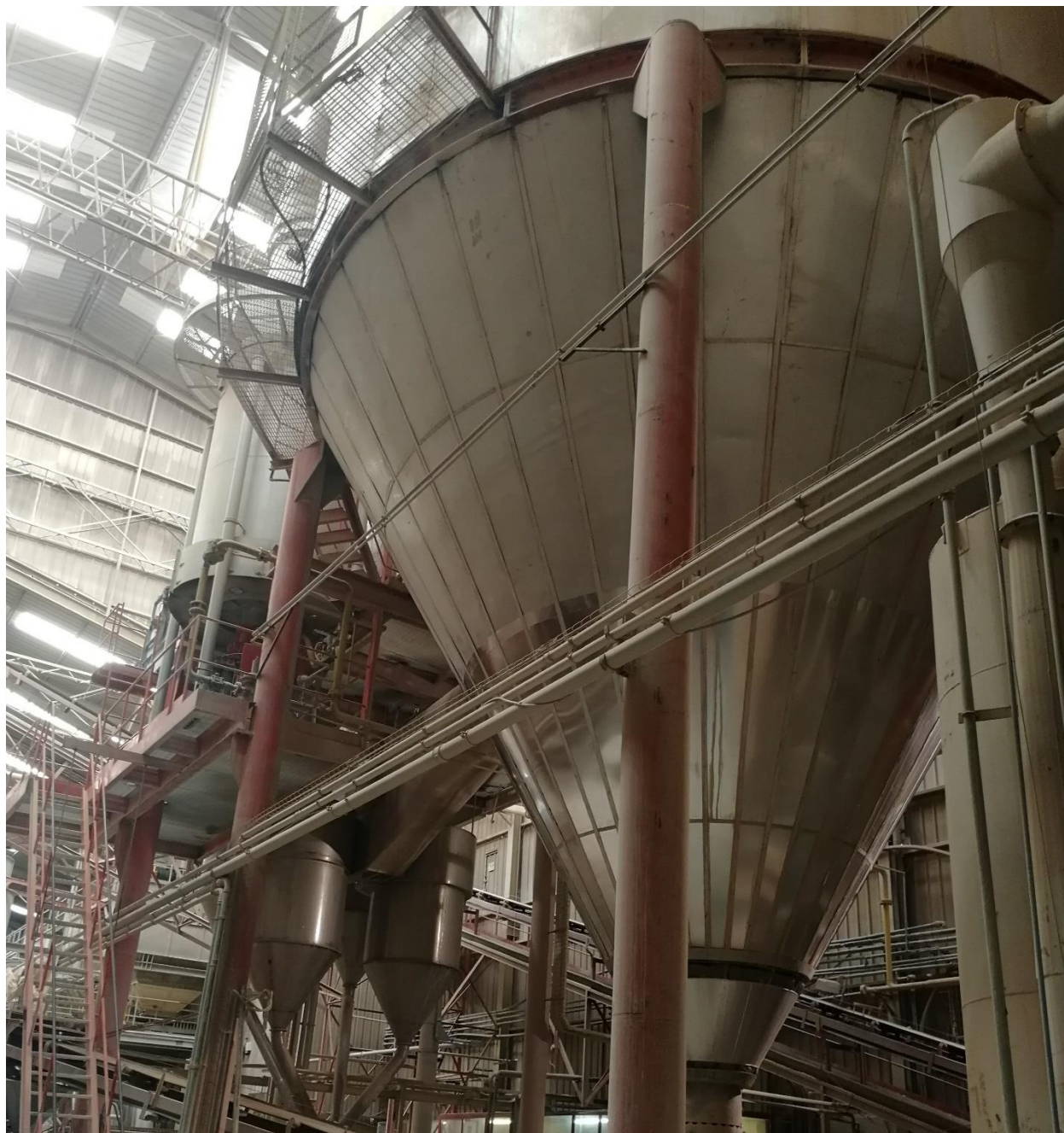
Figure 1.3 - General view of preparation unit
