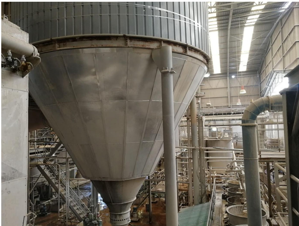
Figure 1.3 - General view of preparation unit
