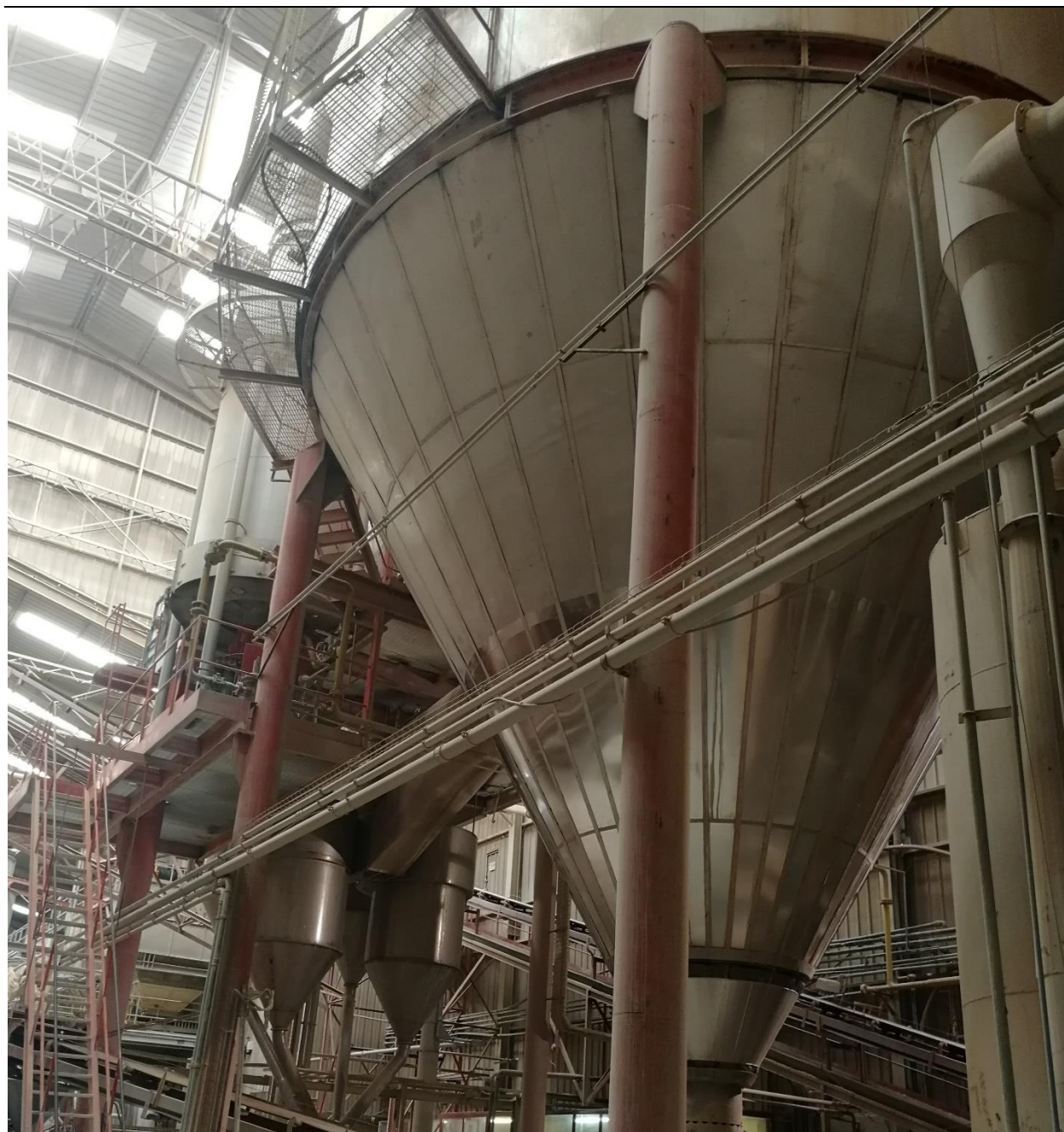
Figure 1.3 - General view of preparation unit
